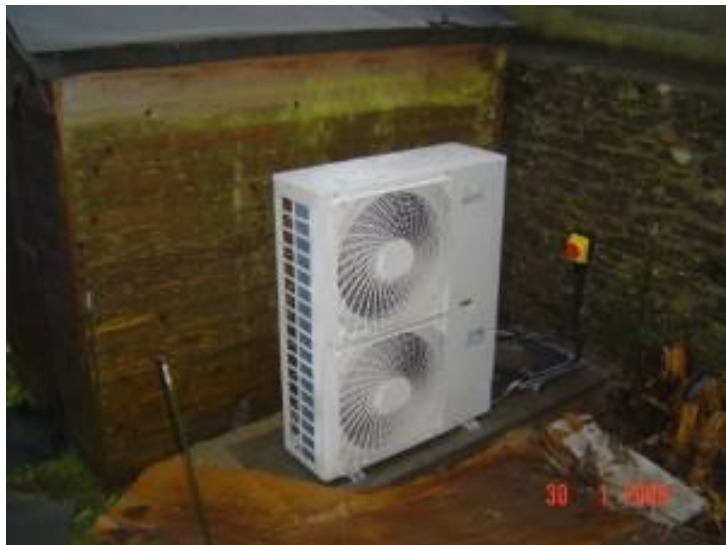
Air source heat pump
